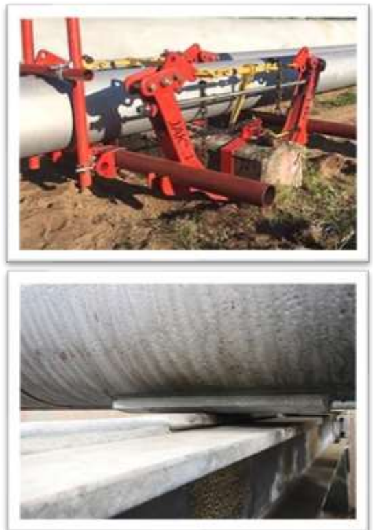
Figure 4: Shows the bare metal finish and pipe support.
