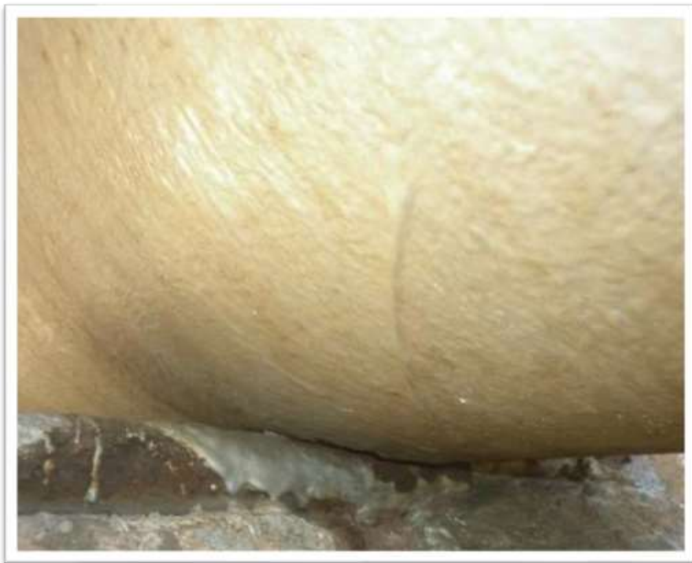
Figure 1: showing the underside of the pipe with external coating yet to be removed, pipe support can be seen under the pipe
