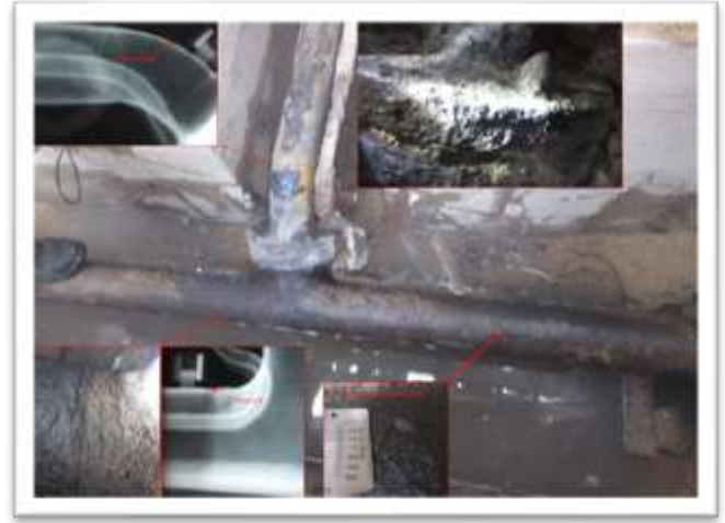
Figure 2: Severe external corrosion of the pipe and flange.
