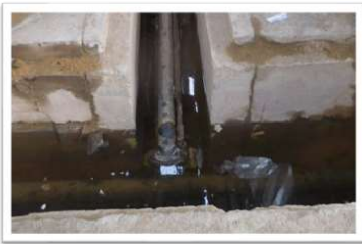
Figure 1: Active leak caused submersion of the pipe and flange.
