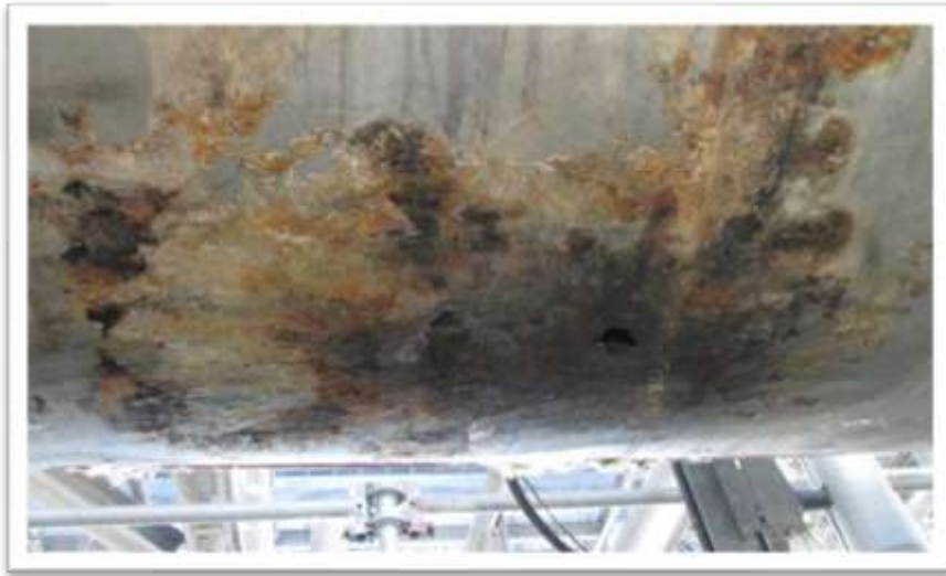
Figure 1: Through wall defect
