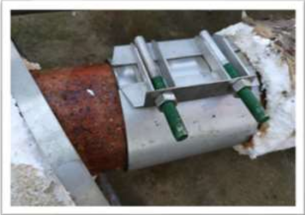
Figure 1: Failed clamp Repair 1
