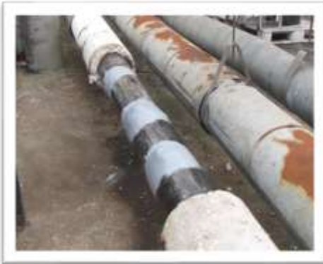
Figure 3: Leaks clamped with straps and profiled with Revofill
