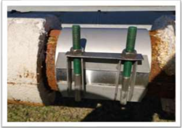
Figure 2: Failed clamp repair 2
