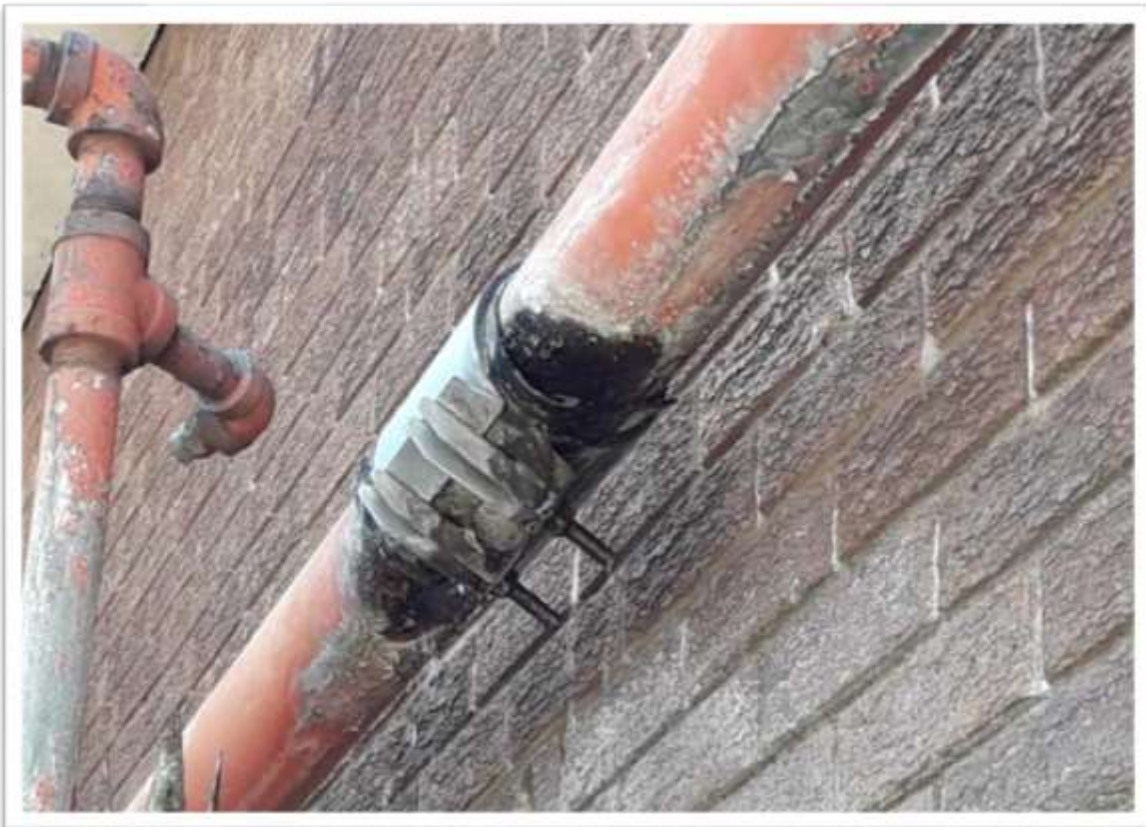
Figure 1: Failed sleeve clamp
