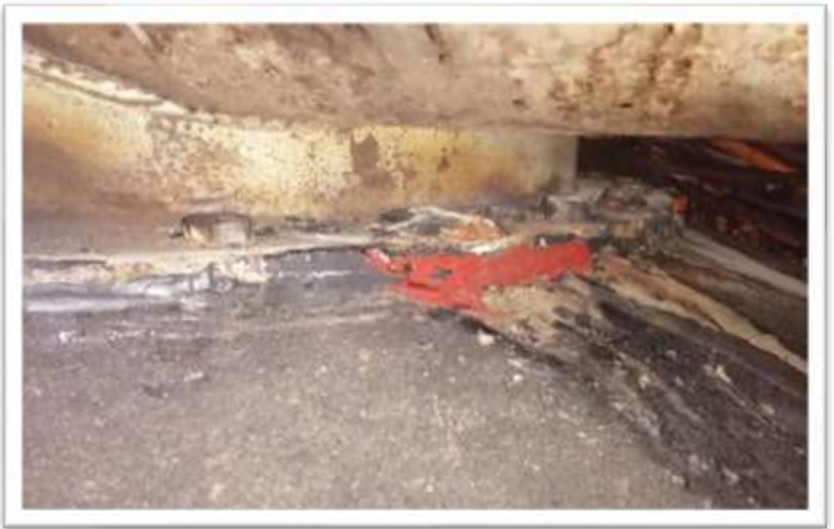
Figure 2: Leak on flanged area
