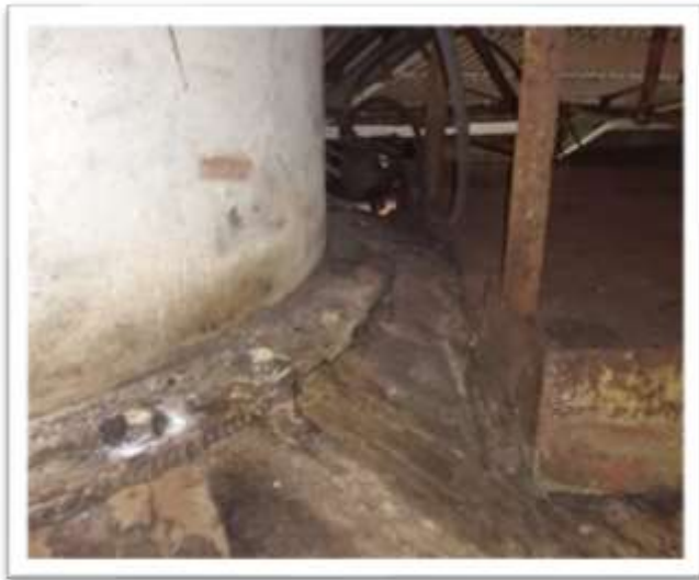
Figure 1: Leak on flanged area
