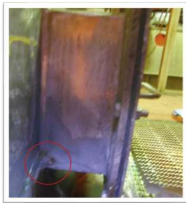
Figure 1 showing manhole with leak
